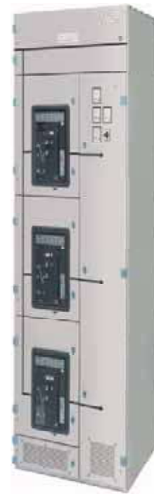
Circuit Breaker Maintain Position
