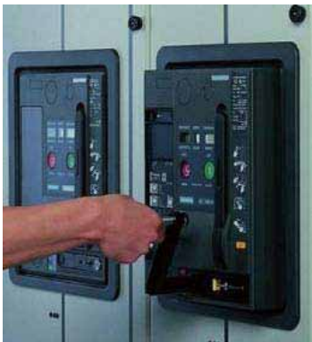
CIRCUIT Breaker DOOR Closed PIX
