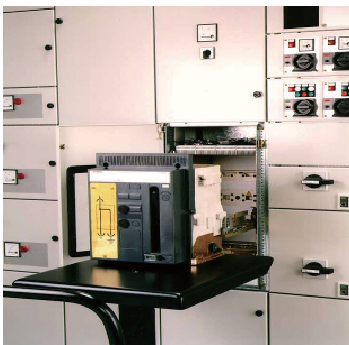
Circuit Breaker Cabinet 6
