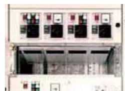
withdrawable module 1, 2, + withdrawable cabinet empty
