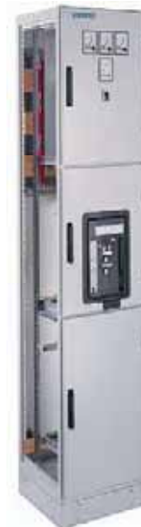
Circuit Breaker Cabinet 2
